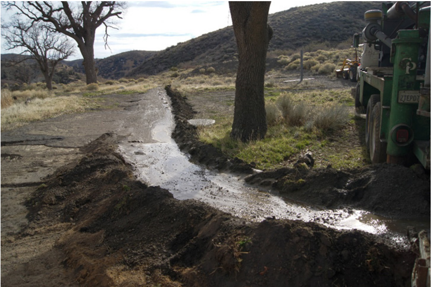
Water flow discharged in trench. Estimated output of water is 800 gallons plus per minute. Unable to drill borehole beyond 65 feet due to large volume of discharged water and debris/cuttings.
